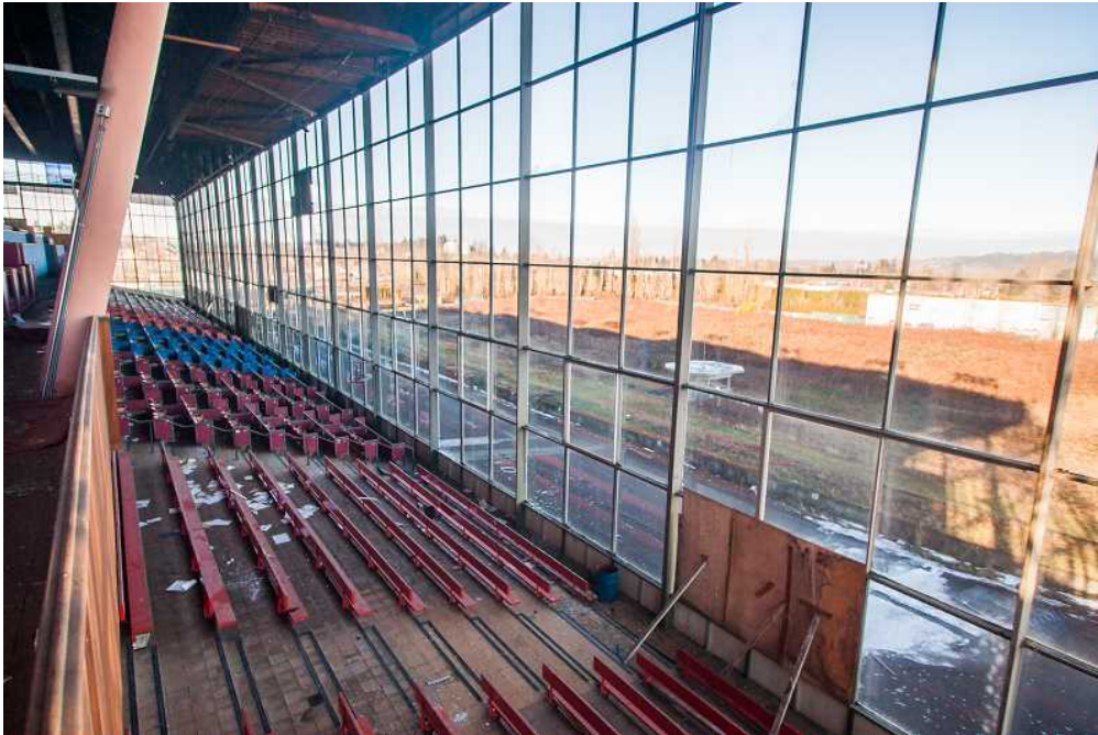
OUTLOOK PHOTO: JOSH KULLA - Today, the grandstand is neglected and filled with debris from the last races held in 2004.
